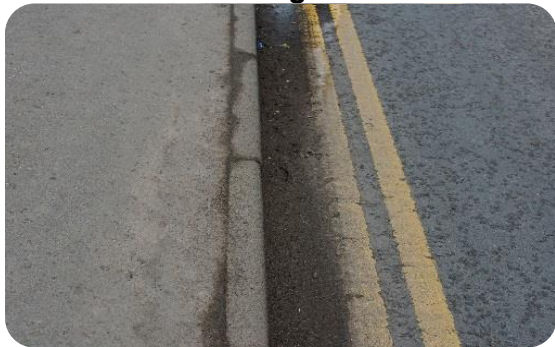
Grade C A significant presence of detritus on roads and gullies
