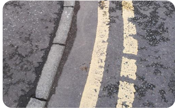
Grade B A slight presence of detritus on roads and gullies
